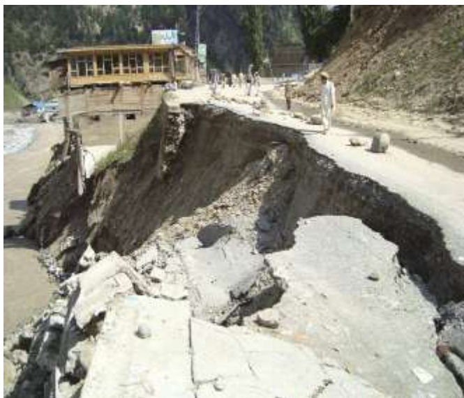
Damaged Road and Hotel in Swat
