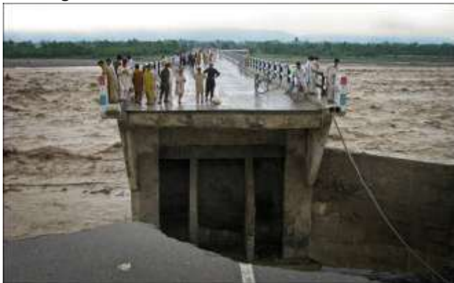
Charsadda Bridge washed away by flashing flood
